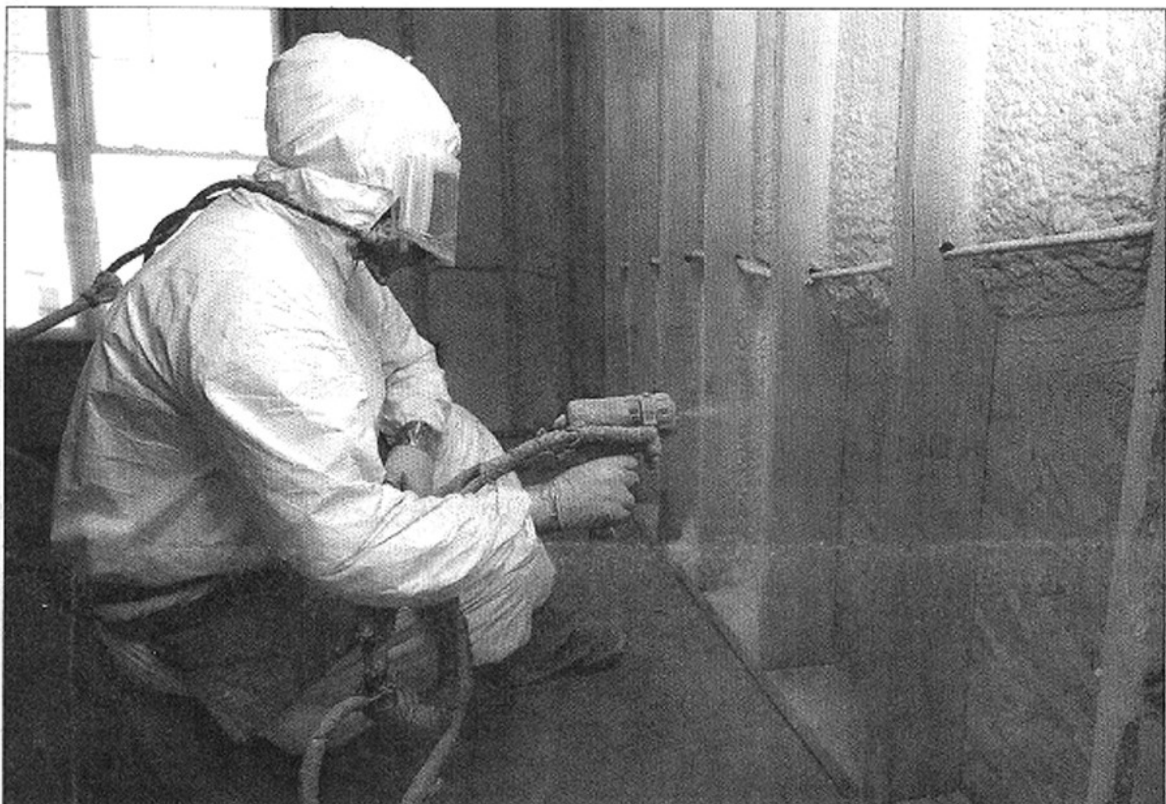
Luis Sanchez of Fairfield Insulation sprays foam insulation into the walls of a home under construction in New Milford. David W. Harple/Staff photographer
