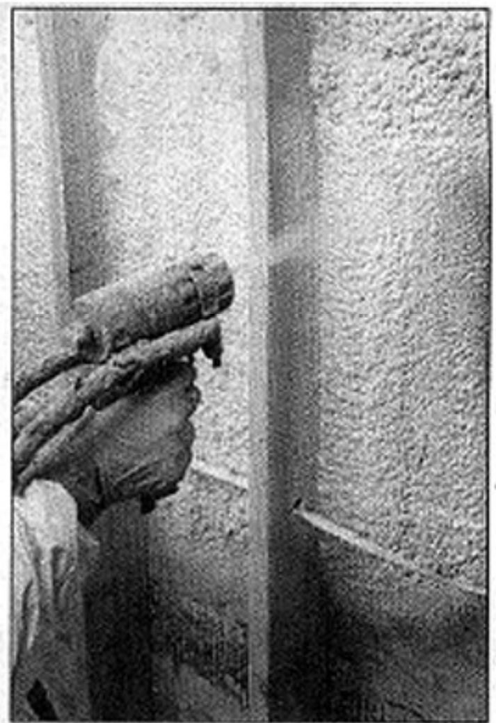
David W. Harple/Staff photographer Foam insulation is sprayed onto the interior walls of a new house in New Milford on Tuesday.
